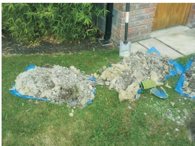
Attic insulation previously placed above 100mm piping dug up as part of trial hole
