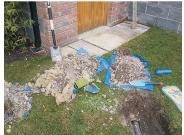
Attic insulation previously placed above 100mm piping dug up as part of trial hole
