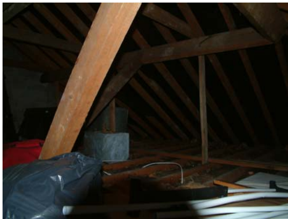
Quilt insulation and old disconnected steel cold water tanks visible in attic space
