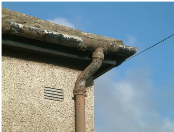
Timber fascias and soffits and cast iron rainwater goods in poor/reasonable condition.
