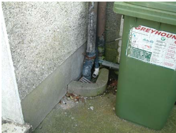
Cast iron rainwater goods in poor condition.
