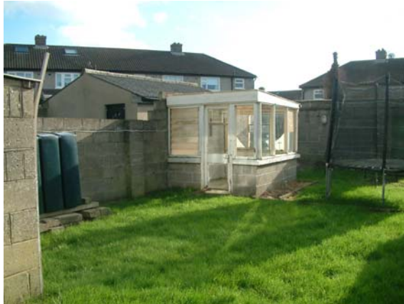
Outbuildings 2 – middle of garden - Flat-roofed conservatory in poor repair)
