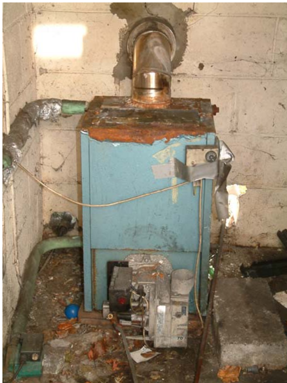
Old kerosene fired heating system located in outhouse at rear of dwelling
