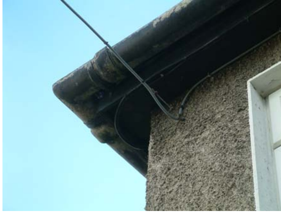
Timber fascias and soffits and cast iron rainwater goods in poor/reasonable condition.
