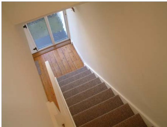
Timber floor finish to hall, and carpet to stairs all in poor condition
