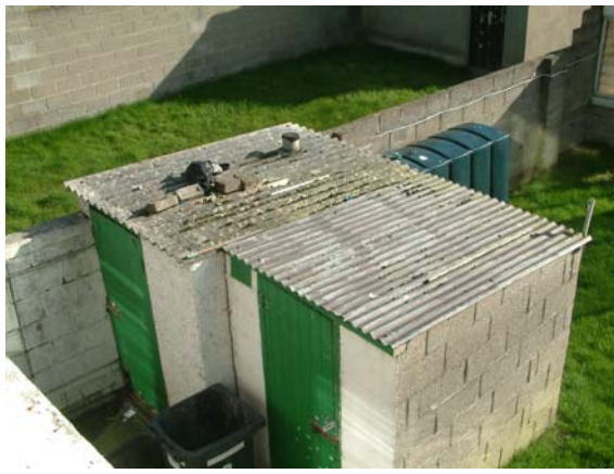
Outbuildings 1 immediately to rear of dwelling with asbestos roofing to boiler house (to be removed as part of any outbuilding renovation)
