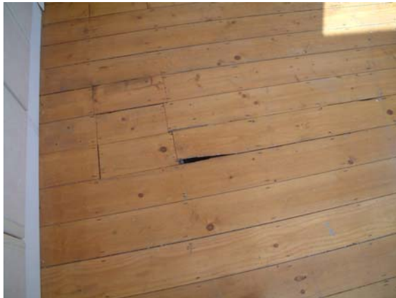
Floors have been stained and varnished throughout, and are in a poor state of repair with some holes evident, flooring having been damaged with prior renovation/heating system work.
