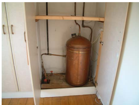
Old un-insulated hot water cylinder in double bedroom to rear.
