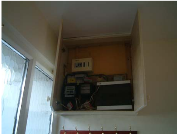
E.S.B. meter & E.L.C.B. board located In wall press adjacent to front door.
