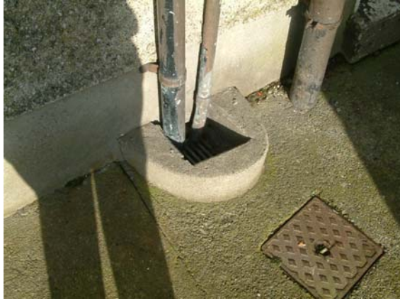
Surface water drainage from rain water pipes to Armstrong junction.
