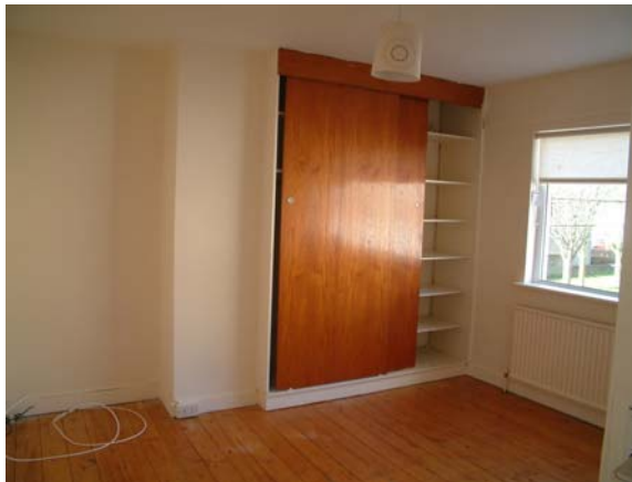
Double bedroom fitted unit in poor condition
