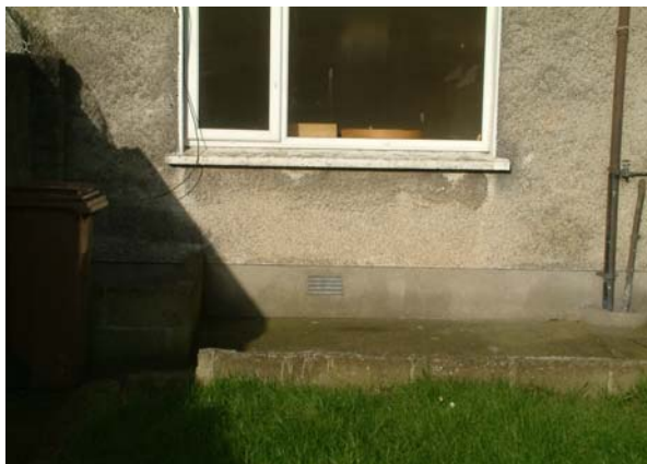
Dashed walls to rear elevation with underfloor room vent visible to ensure circulation of air under raised timber floor.
