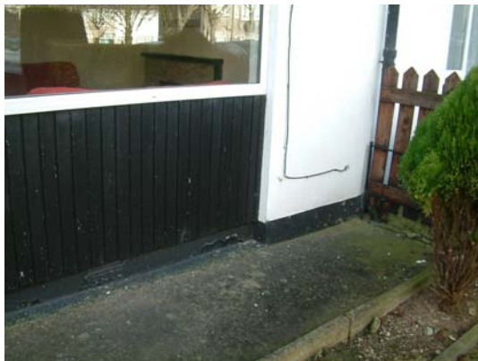
Timber panelling in poor/reasonable condition beneath front living room window, and loose cabling running through large hole in wall
