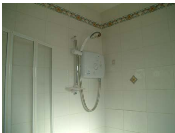
Bathroom tiling in poor repair with pumped electric shower installed (Triton T90)
