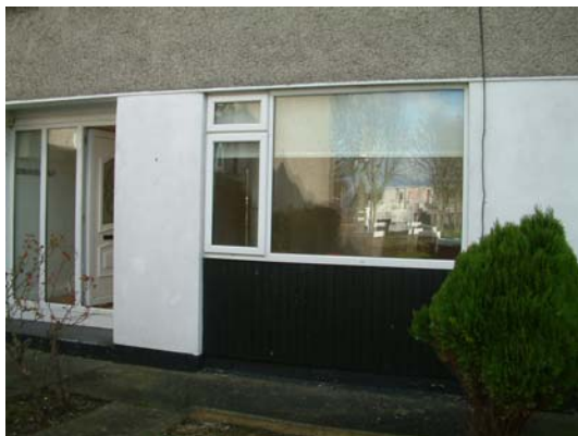
Upvc Double glazed window and front hall doorset with badly fitting opening sections
