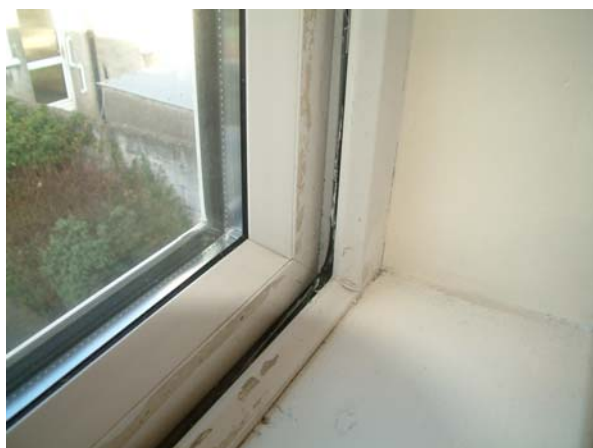
Badly fitting windows with evidence of flexible sealant being used to (badly)draught-proof the opening sections
