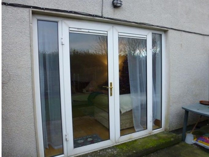
Rear doorset in reasonable condition
