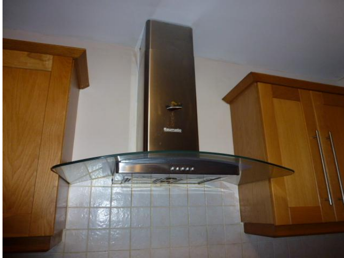
Mechanical vent to kitchen
