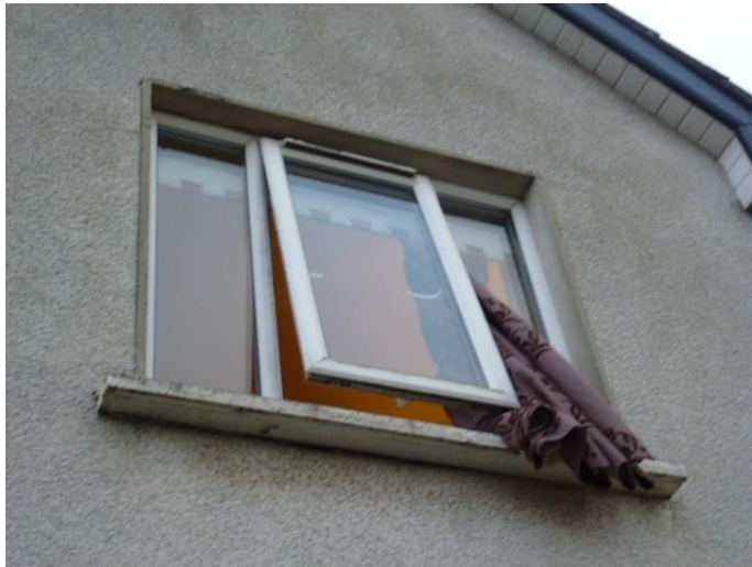
Rear windows in reasonable condition
