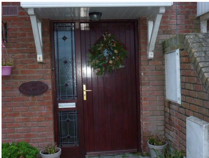
Front doorset in reasonable condition
