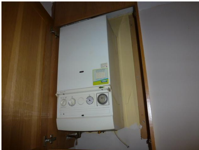
boiler in kitchen unit
