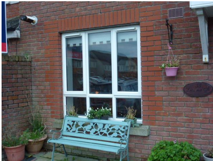
Front windows in reasonable condition
